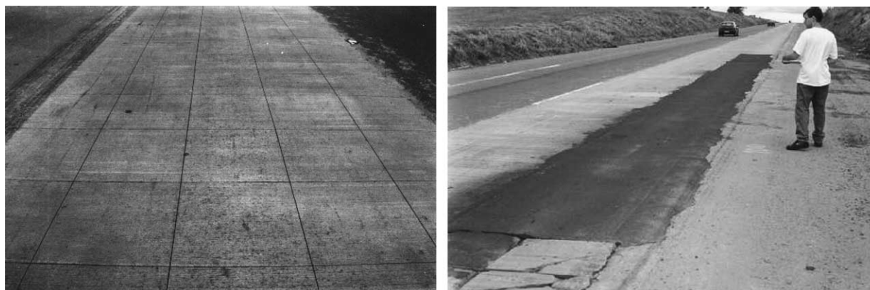
Figure 4. UTW at SP-280 test sections as constructed (left) and after 3 months (right).
